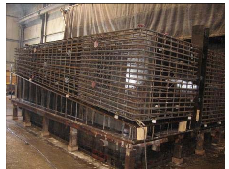
Cage is secured on the pallet, spaced to the core, awaiting jacket closure and concrete pour.
