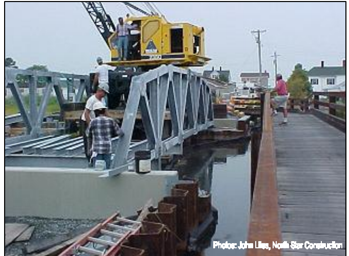
Specially designed superstructure placed on precast abutments with pre-welded stainless steel reinforcement.
